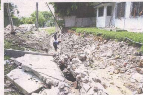
The debris of a collapsed retention wall of a home in Taman Ukay Heights following a mudflow on Nov 11. — Filepic
